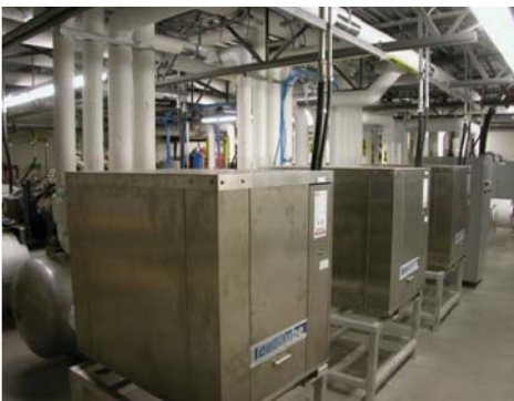
Central heat pumps
